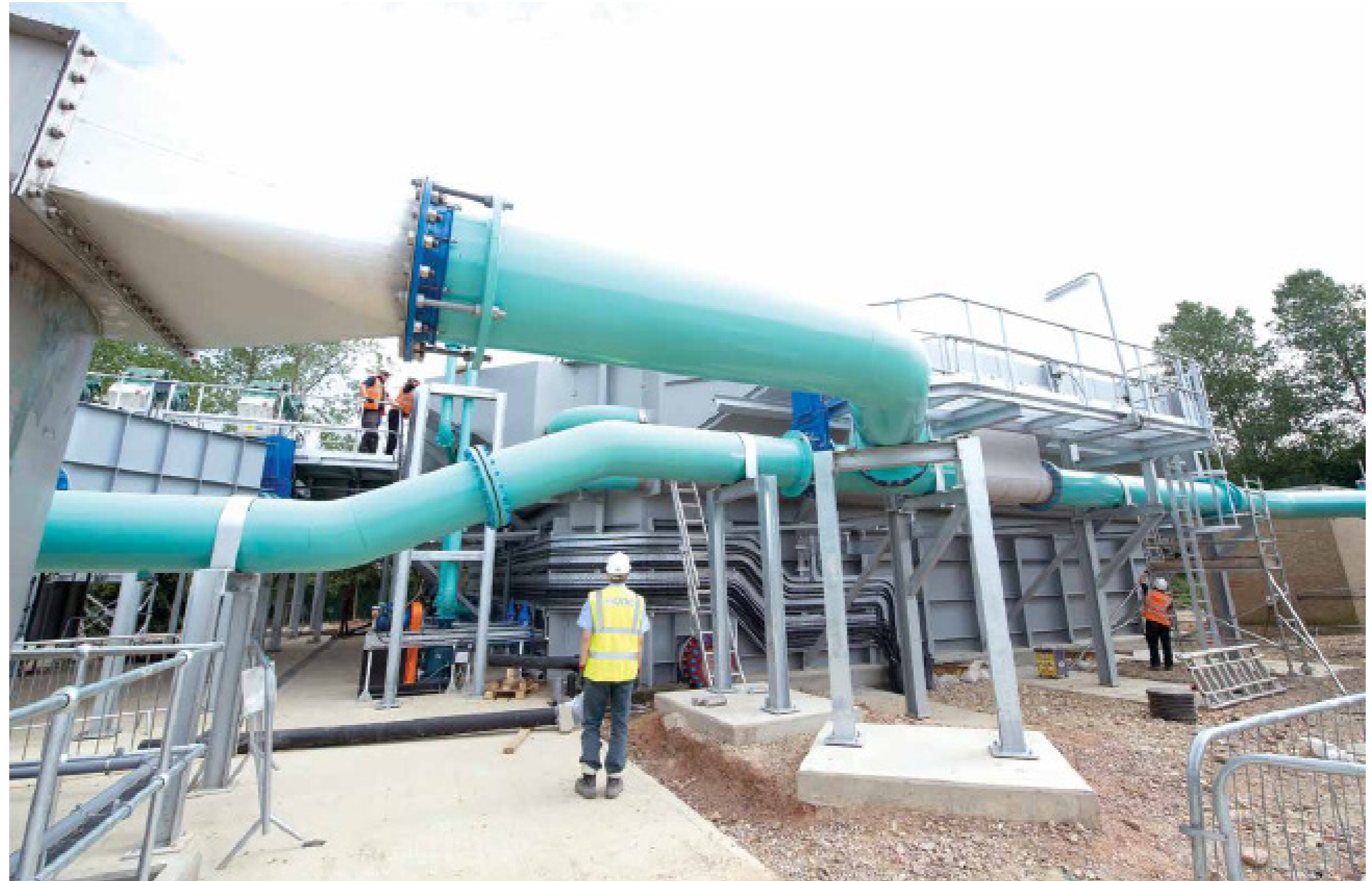
Storm Surge and Balancing Tanks (background), Hydro Grit King hydrodynamic vortex separator (left). Raw water intake is a mixture of combined sewers, dedicated foul water sewers and commercial waste water. On low flow volume days all inlet water is processed through the Grit King. During storm days a proportion of water is diverted to the storm tank for settling.
