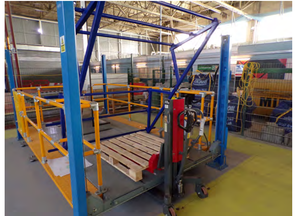
Modified car lifting jack, used to create a safe working platform for operatives stacking Superblocks - see Sub Assembly case study
